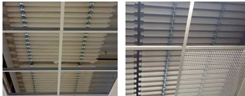
Figure 4. Phase change materials tubes (Final Installation on-site)
